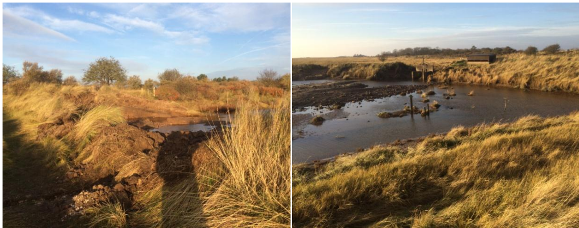
Breach point in Bulldog Bank Sluce
